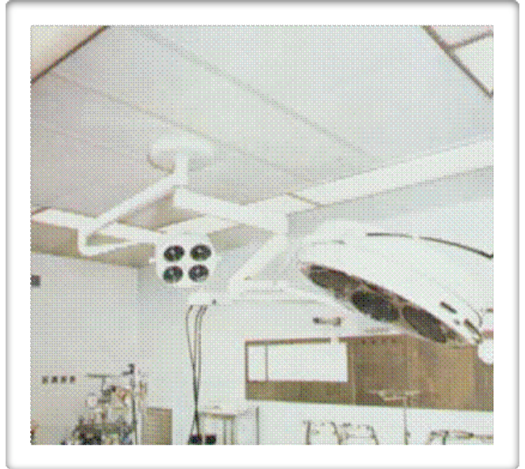
Typical installation of Laminar Flow Panels
